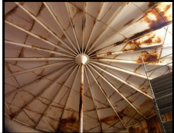
Figure 10; Interior Tank Damage
